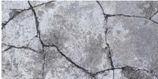
Above: Severely distressed concrete
