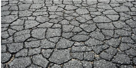
Above: Severely distressed asphalt
